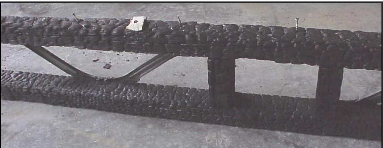
Photograph 10. The same joist as above.
